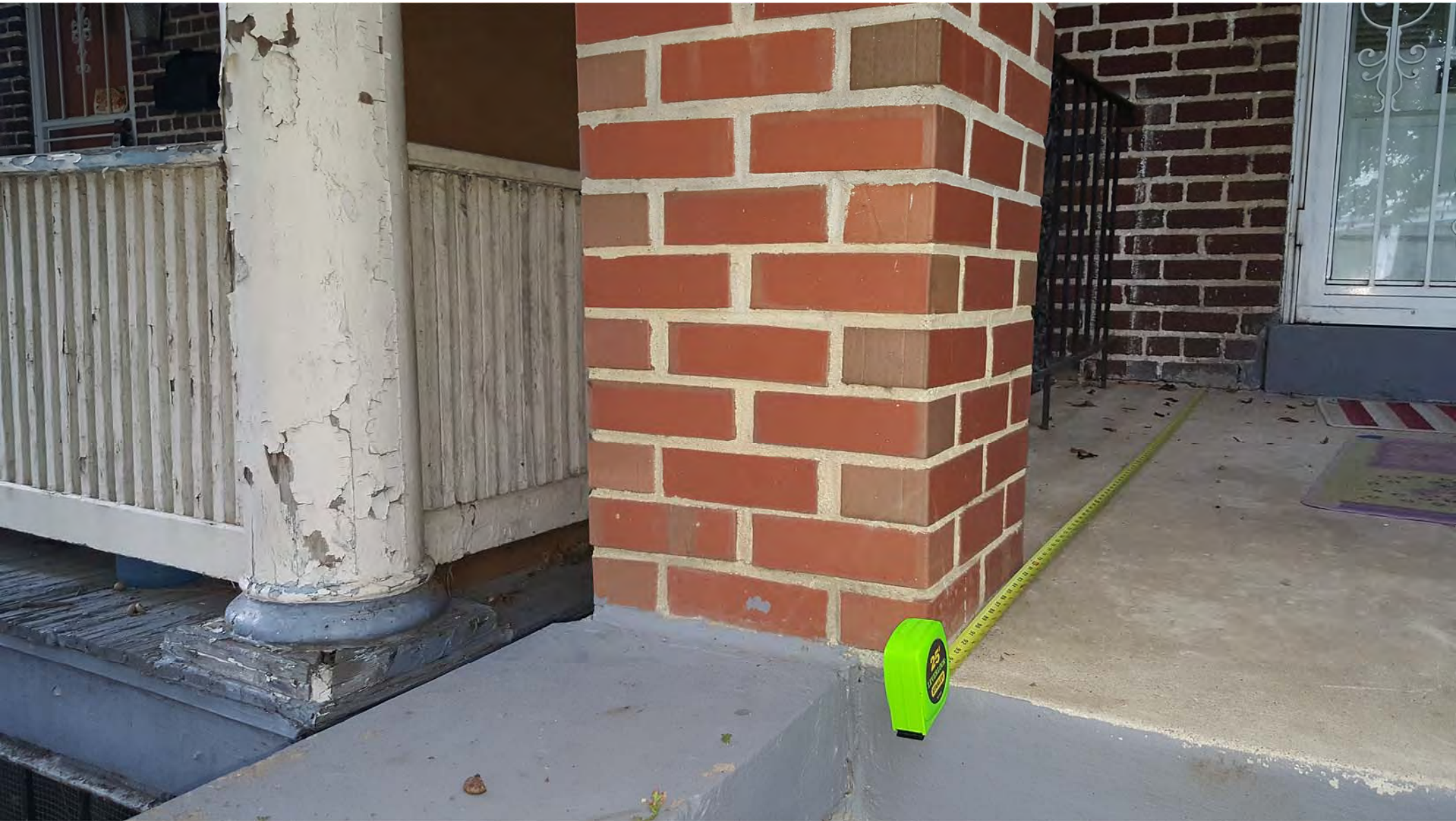
Subject Property to the left, 1115 Allison to the right (with tape measure)
